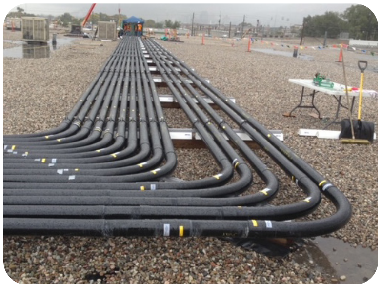
Exposed conduit is subject to environmental factors such as temperature, humidity, precipitation and pollutants that cause corrosion.
