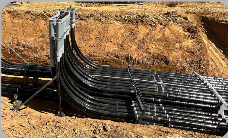
Buried conduit can be subject to stress corrosion cracking which can damage conduit systems.
