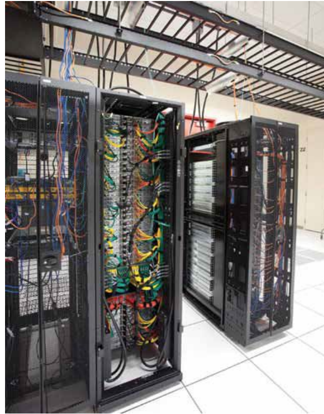
Figure 1: Increasing demand for cloud services is putting a strain on server capacity. This photo shows data center servers while they are being configured and wired. Courtesy: Jacobs Engineering
