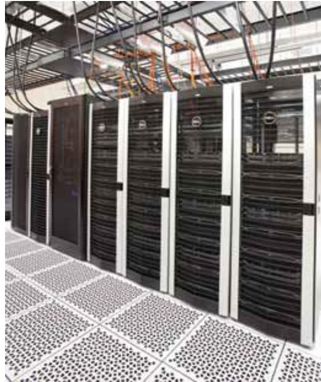
Figure 2: For many years, ac has been the dominating form of data center power distribution as shown in this photo of servers powered through overhead busways via busplugs. Courtesy: Jacobs Engineering
