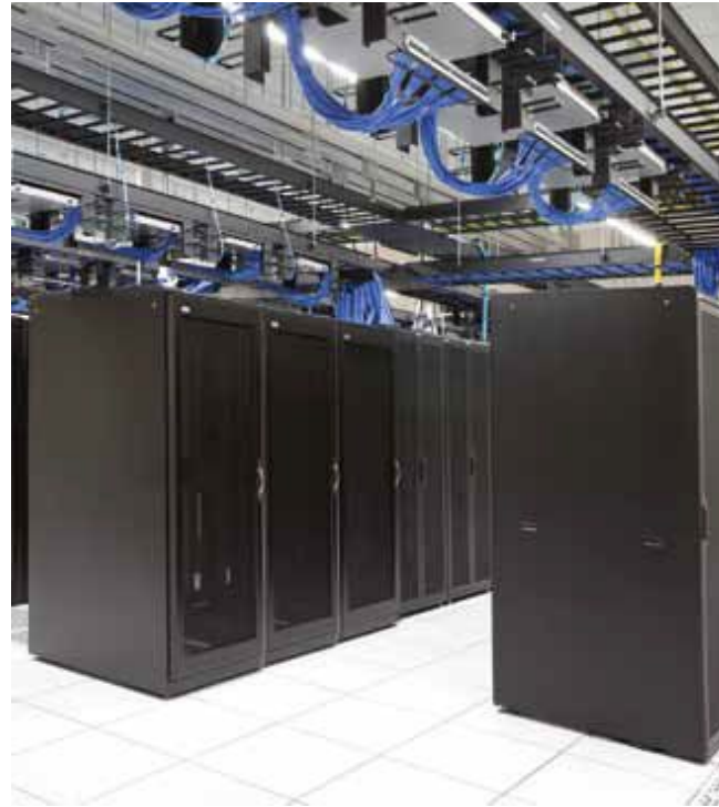
Figure 4: Although data center design can be complex, the completed project can be efficient, reliable, and robust if designed well.
