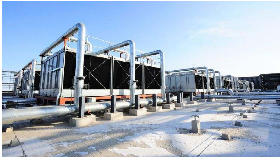
Evaporative cooling towers are an integral part of many data center cooling systems, depending on their location.
