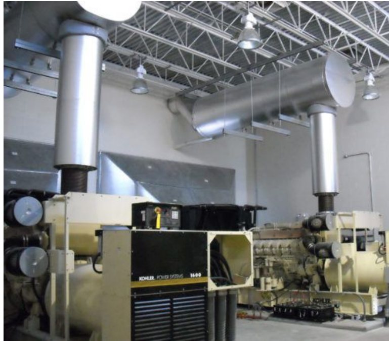
Figure 2: This shows a generator located in a building facing the exhaust side of the space. This image highlights the advantages of a fully customizable space and space for maintenance. Courtesy: CDM Smith
