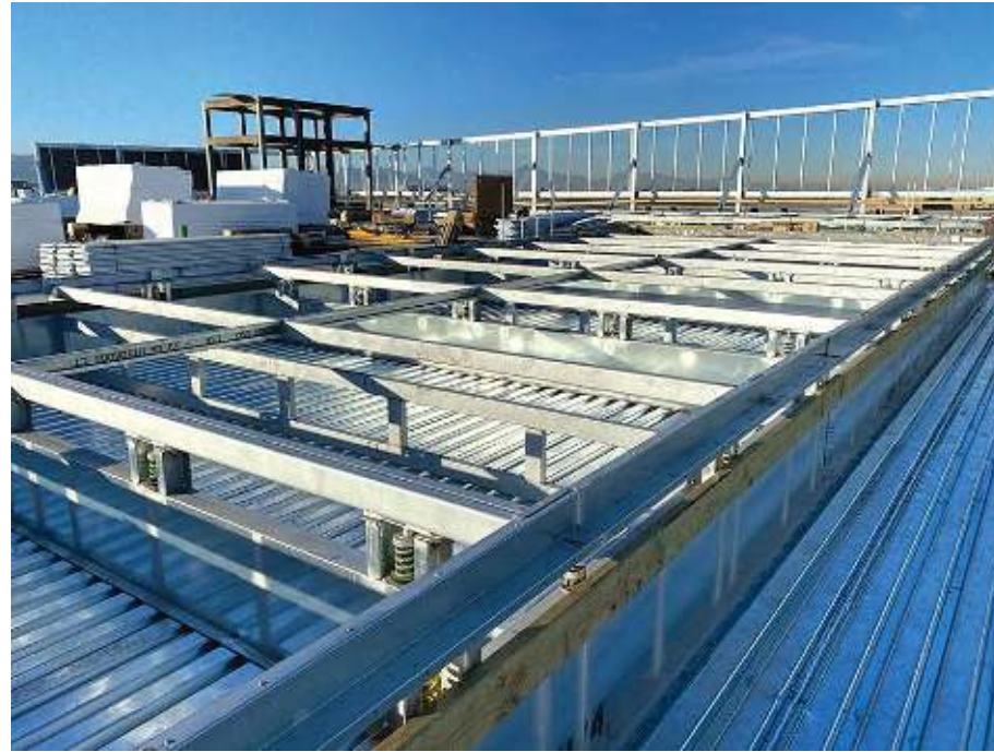
Figure 4: A vibration curb is used to isolate a rooftop unit from transmitting sound and vibrations to the building structure. Courtesy: SmithGroup
