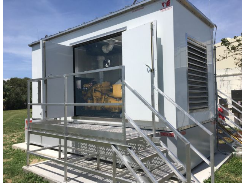
Figure 3: Shown is a generator located in outdoor enclosure with sub-base fuel tank. This image highlights the small site footprint of an outdoor enclosure and the limited amount of space around and within the enclosure for maintenance.
