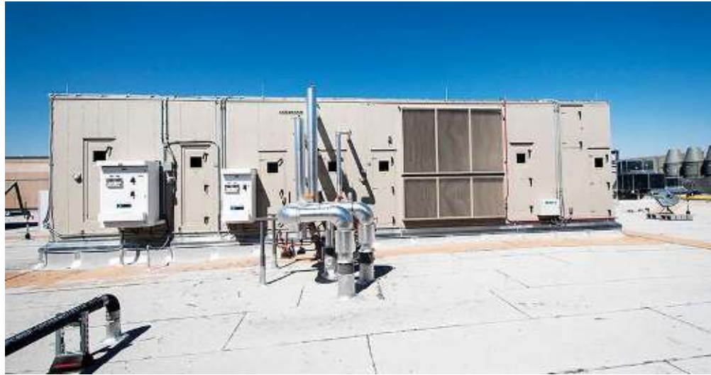
Figure 2: An applied rooftop unit has multiple coils and airside economizer. Courtesy: SmithGroup/Liam Fredrick
