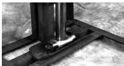
For high-impact, steel conduit will collapse and can pinch the cable. This will make repair of damaged conduit more difficult.
